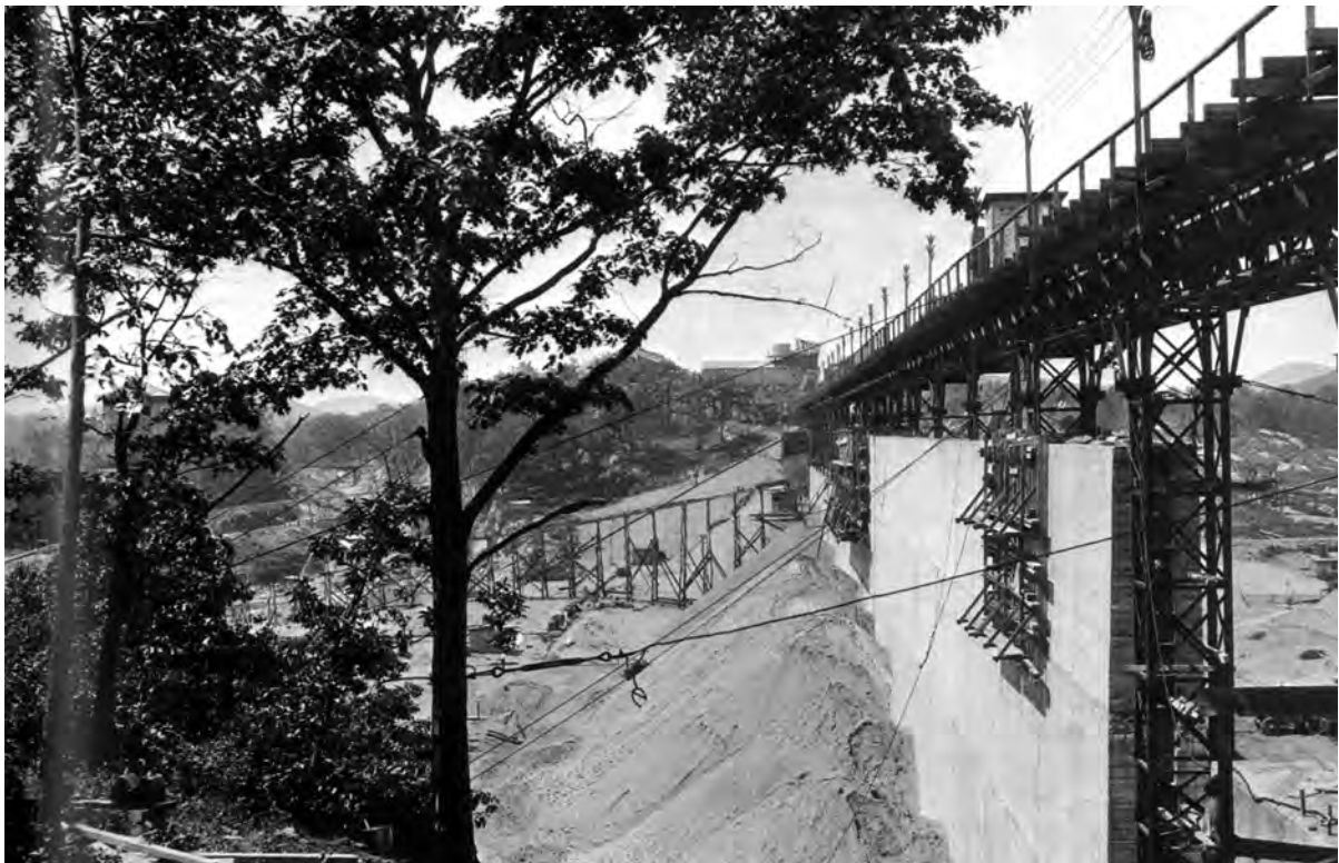
Construction of the Wanaque Reservoir, between 1920 and 1930. Photo taken from Newark, by John Cunningham.
